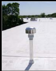
Passive vent pipe
